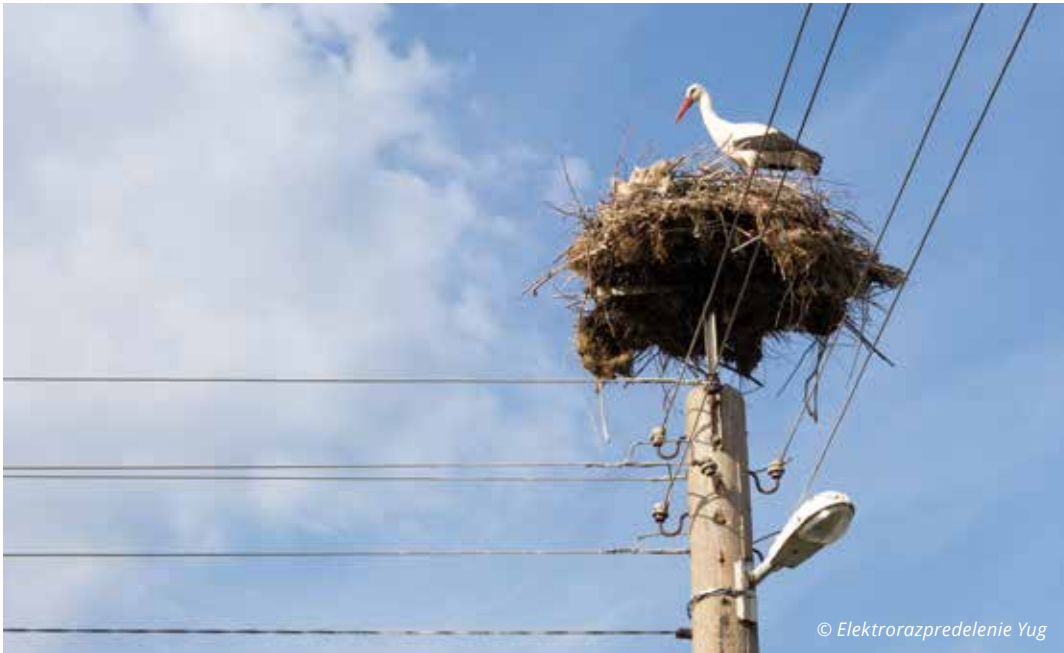
Mounted stork nest platform. The nest is lifted to a safety distance from the conductors
