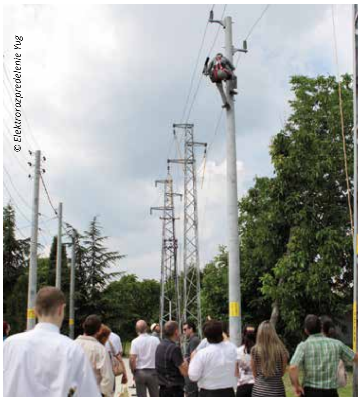
Demonstration – installation of protective insulations on poles. Training area in Stara Zagora, 2014
